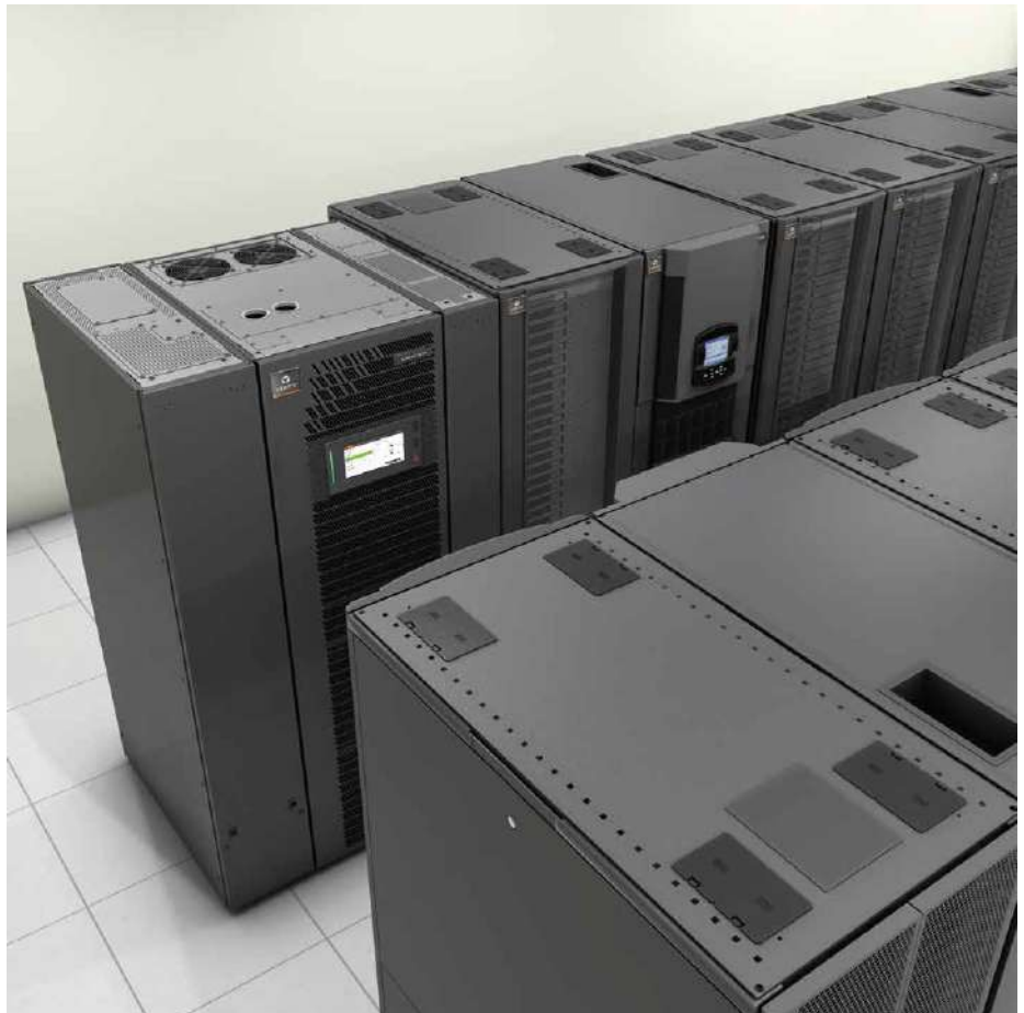
Liebert eXM (160-200 kVA) with switch sidecar
