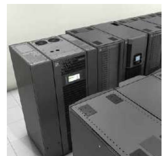
Liebert eXM adjacent to the wall
