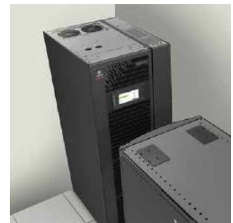
Liebert eXM detached from the wall
